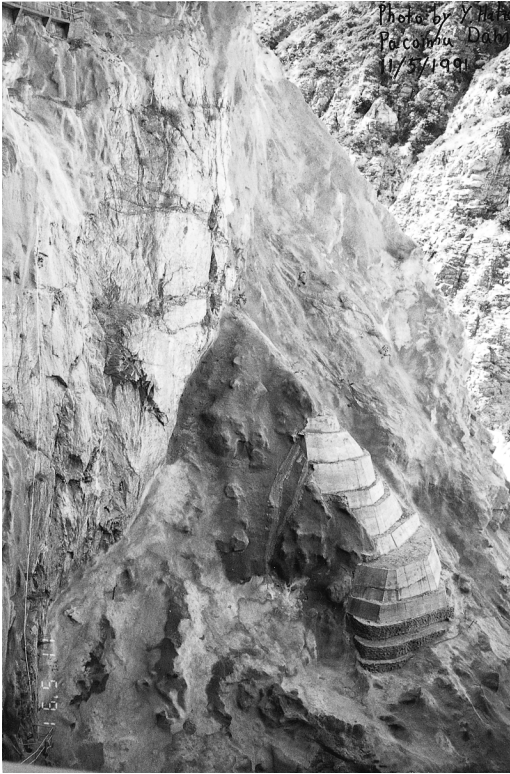
Fig. 14. Site of left abutment failure
