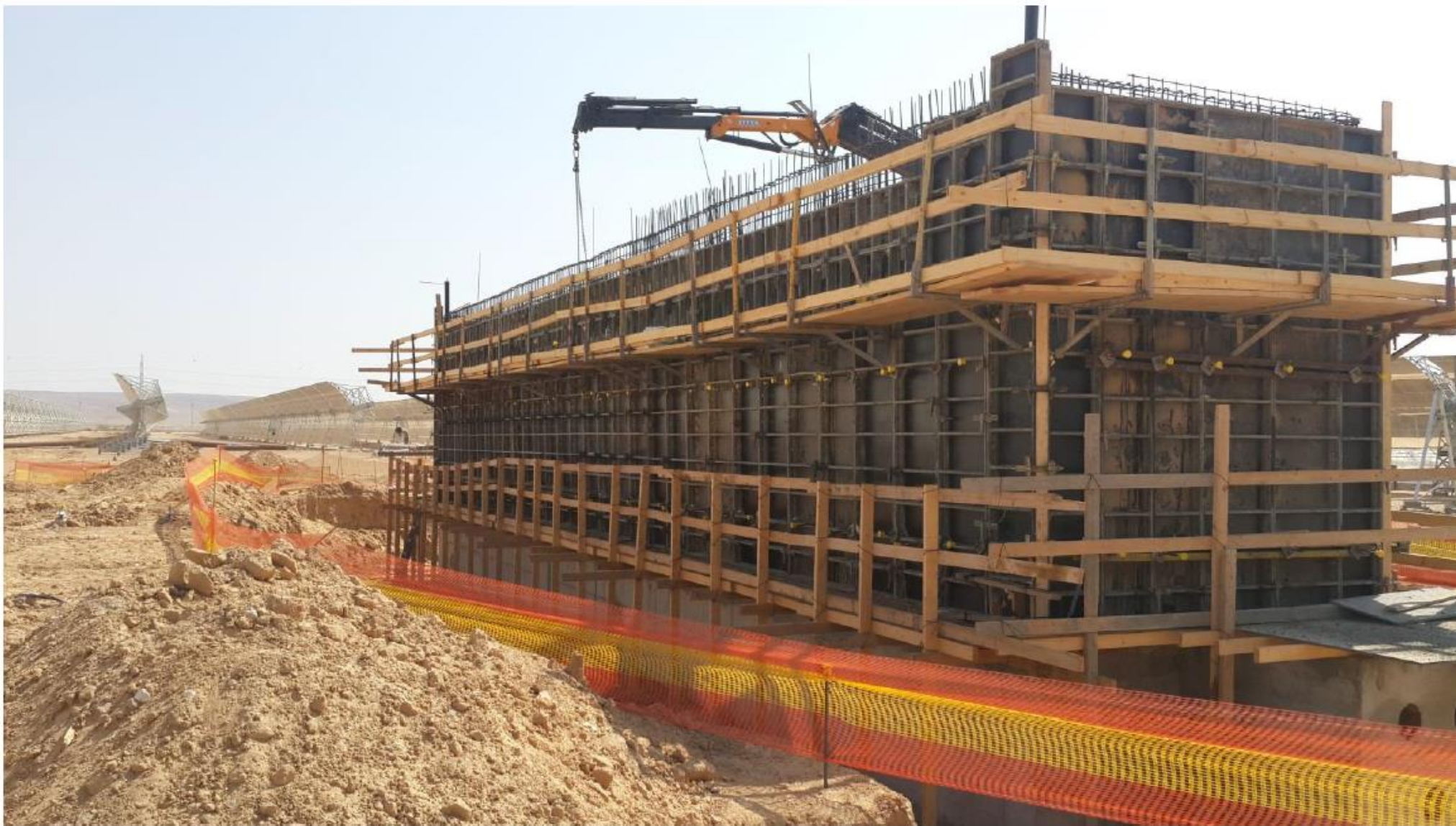
Solar Field Auxiliary Electrical Building No. 1
