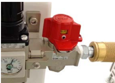
Figure 5: Example of a Red Gas Lockout Valve
