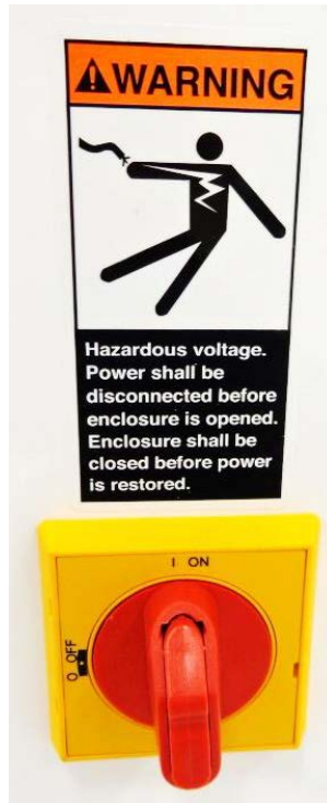
Figure 42: Example of a Main Power Switch
