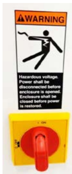
Figure 6: Example of a Main Power Switch
