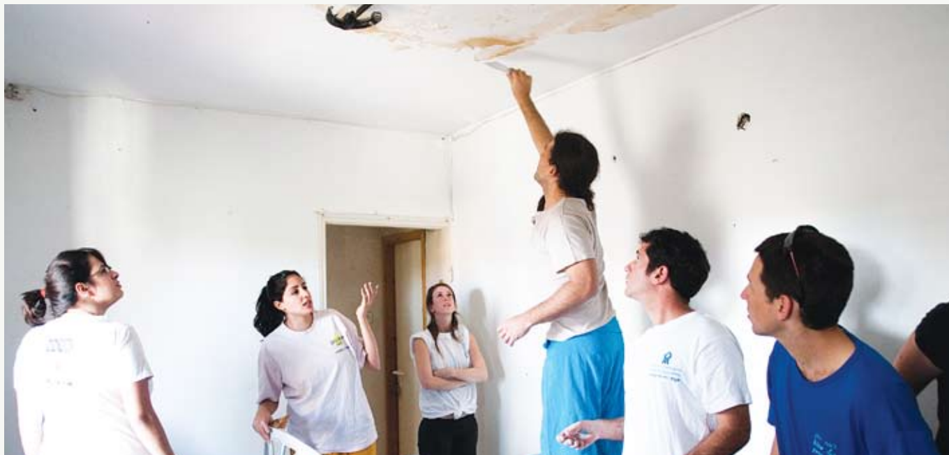
BGU students brought some color into the lives of elderly and needy Beer-Sheva residents by giving their apartments a fresh coat of paint before Passover. The painting activity in low-income neighborhoods was part of the Open Apartments Program in the Community Action Unit
